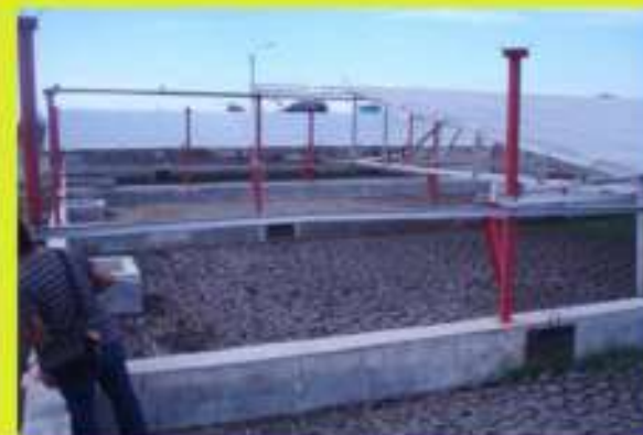
Sledge drying bed – west side – basin 4
