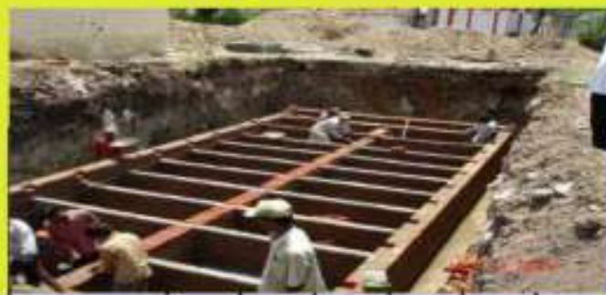
Anaerobic Baffled Reactor
