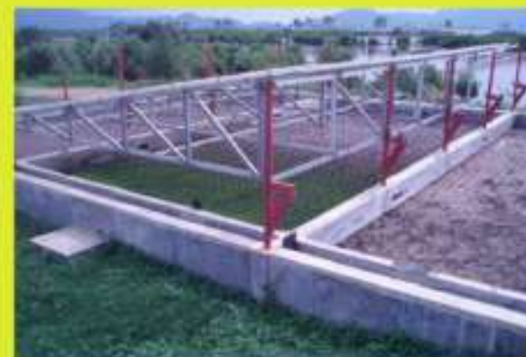
Sledge drying bed – west side – basin 4
